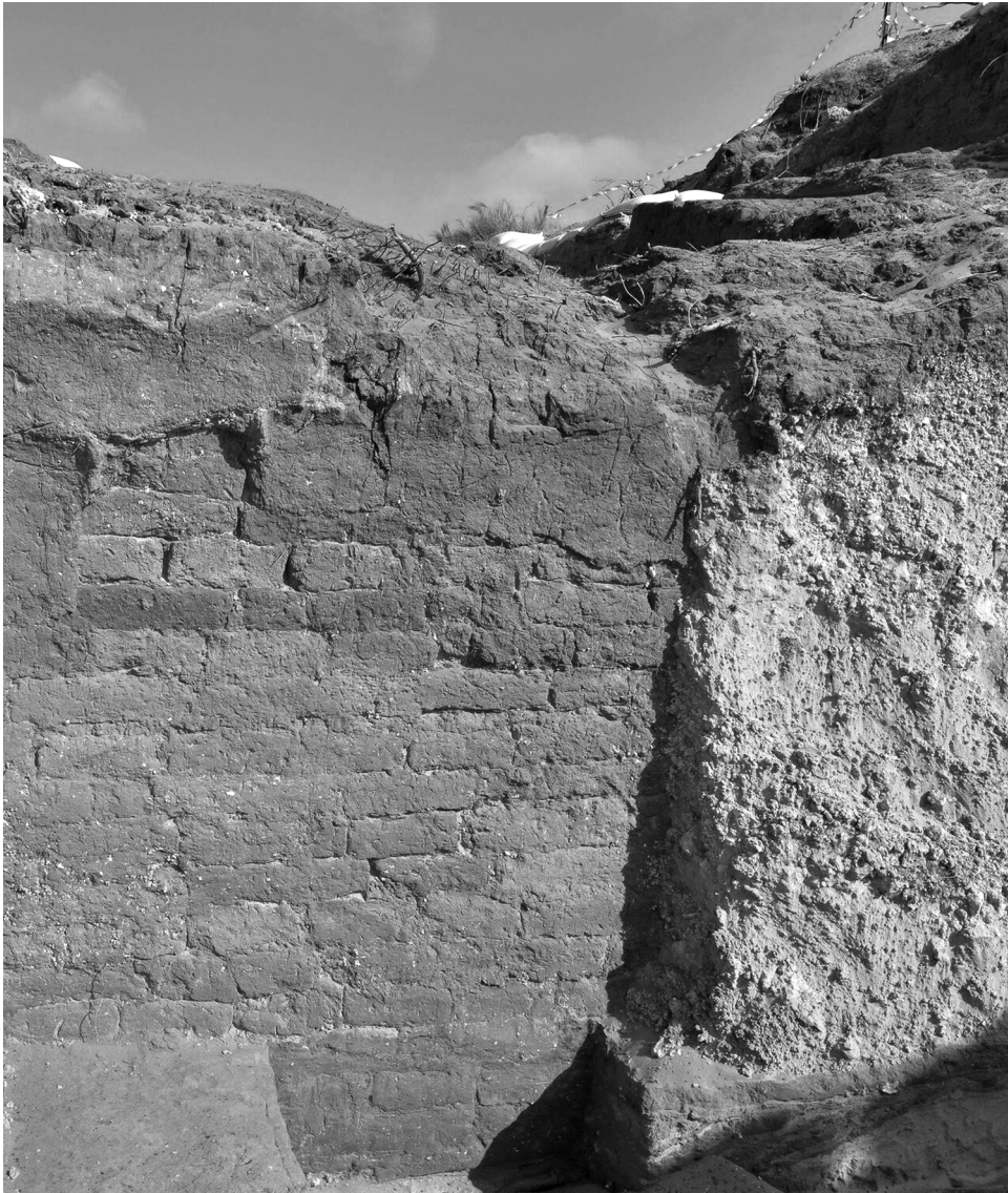
FIGURE 7.5. A close-up of the Iron IIB mud-brick fortification wall (photo by Philip Sapirstein)
